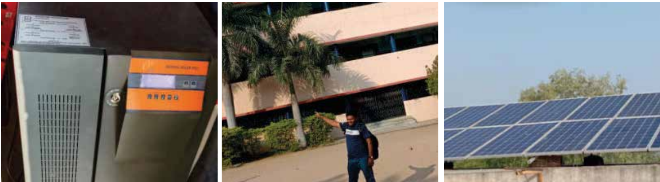
4KVA Off Grid System at District Court Azamgarh
