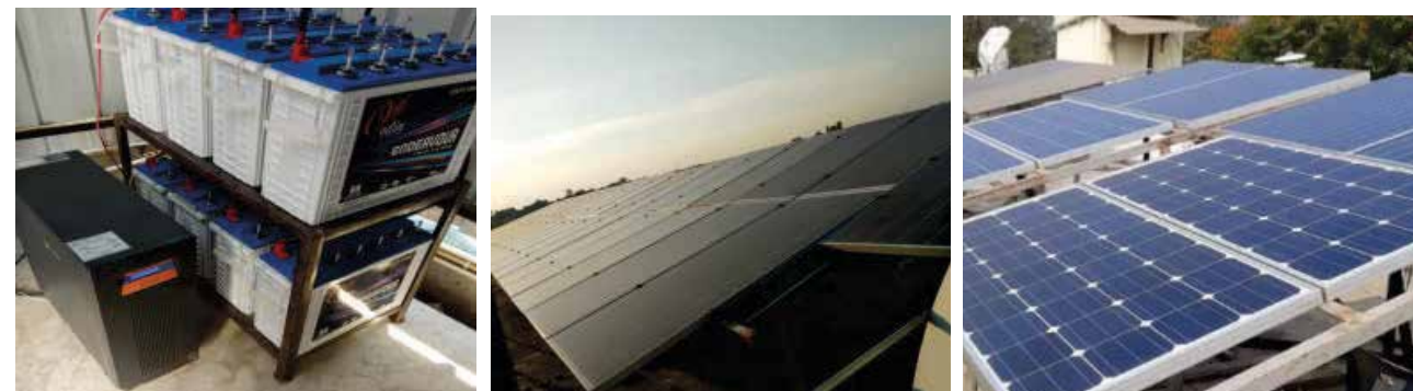
20KVA off-grid Installed at Kanpur
