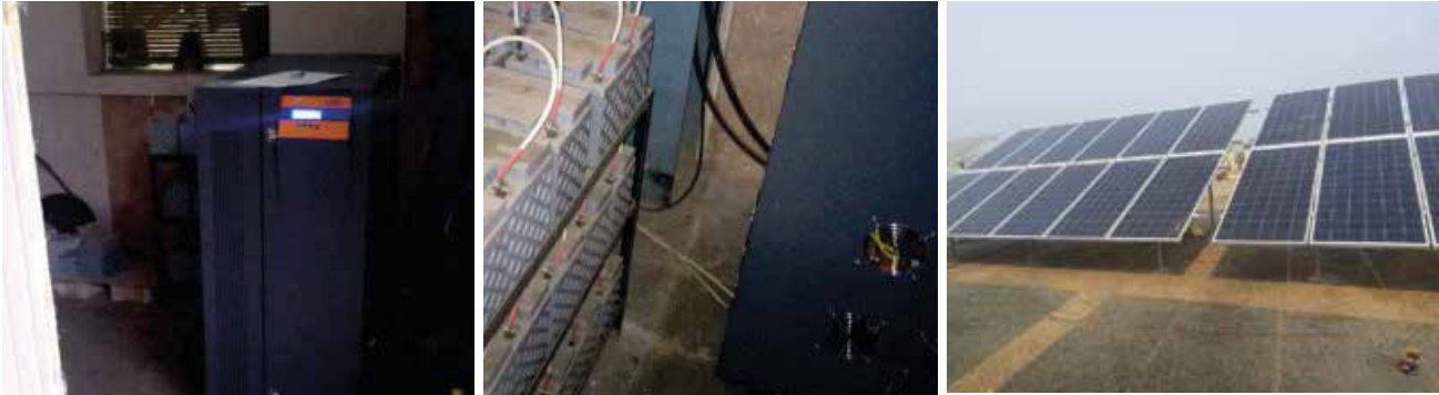
5KVA Off Grid System at Gurgaon
