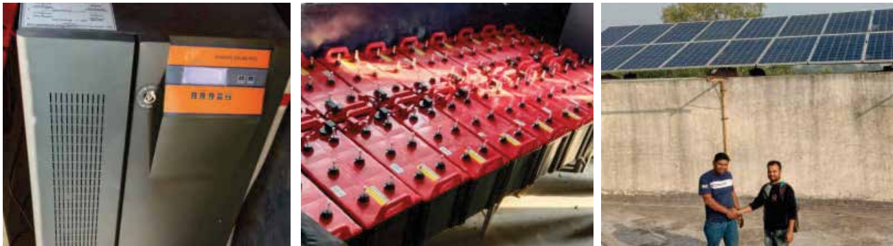
20KVA Off Grid System at BHU Varanasi
