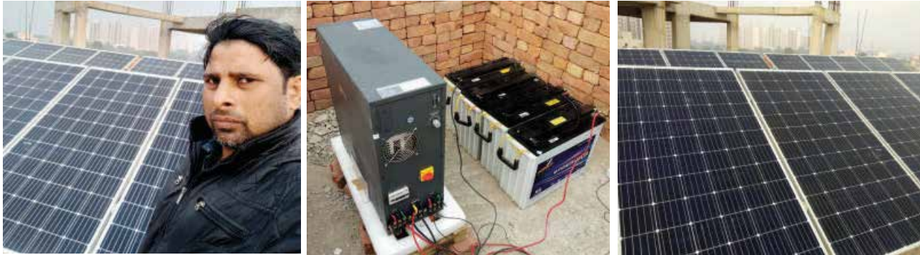
20KVA Off Grid System at Bhopal Engineering college
